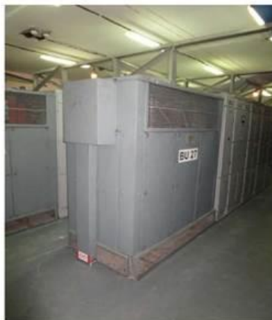
Figure 22. Transformer Component located at Zaporizhzhia Nuclear Power Plant (NPP)
