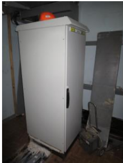
Figure 23. Control Monitor Cabinet located at Zaporizhzhia Nuclear Power Plant (NPP)
